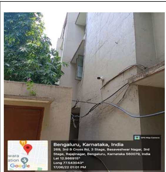
CCTV at the backyard
